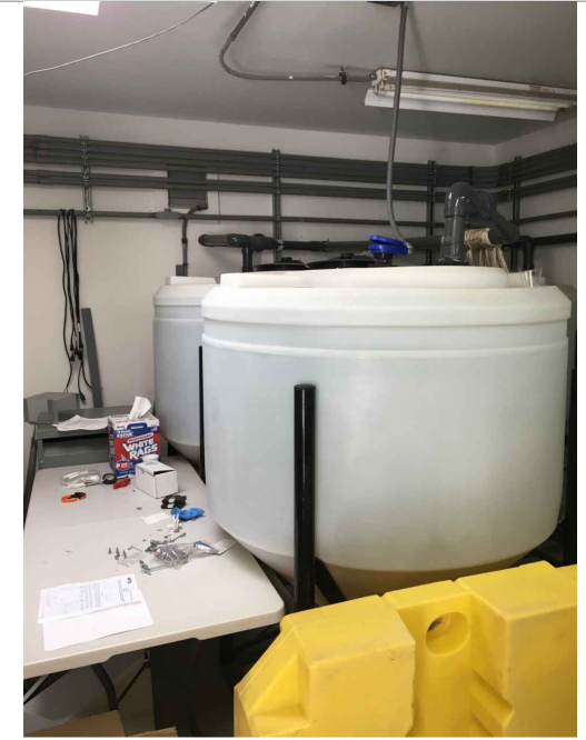
Photo 3 - Forks Treatment Building Interior Figure 1
